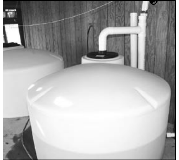
Rainwater collected from the roof of the Wrights' house provides potable water that is stored in four tanks that hold 550 gallons each. The water is run through a regular five-micron filter, available at local hardware stores, and then purified with ultraviolet light from a special bulb. Nature has distilled the water so it's "soft" and requires no treatment to remove iron or minerals. The system costs about $3,000, not including labor. An environmental advantage is that less rainwater washes from the property, so less potential contamination reaches the Bay.
